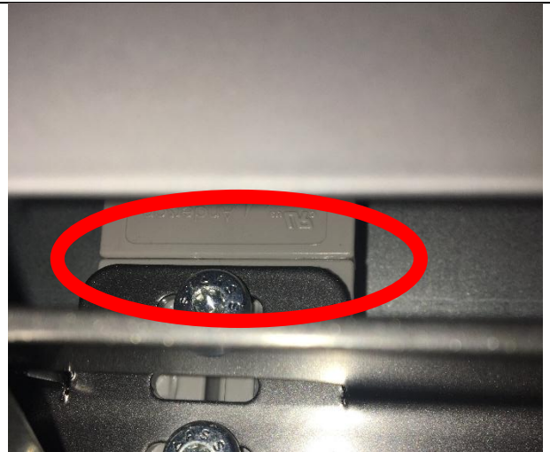
This Photo shows a good connection!
